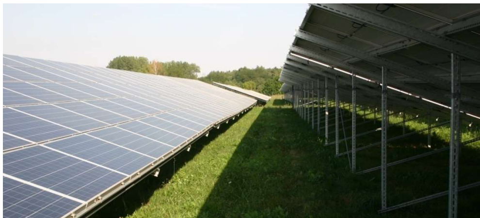
Figure 1-7: Row spacing of about 2.5 metres in a solar farm north of Neuhardenberg (Brandenburg) airfield. Area exposed to sunlight approx. 0.8 m wide
